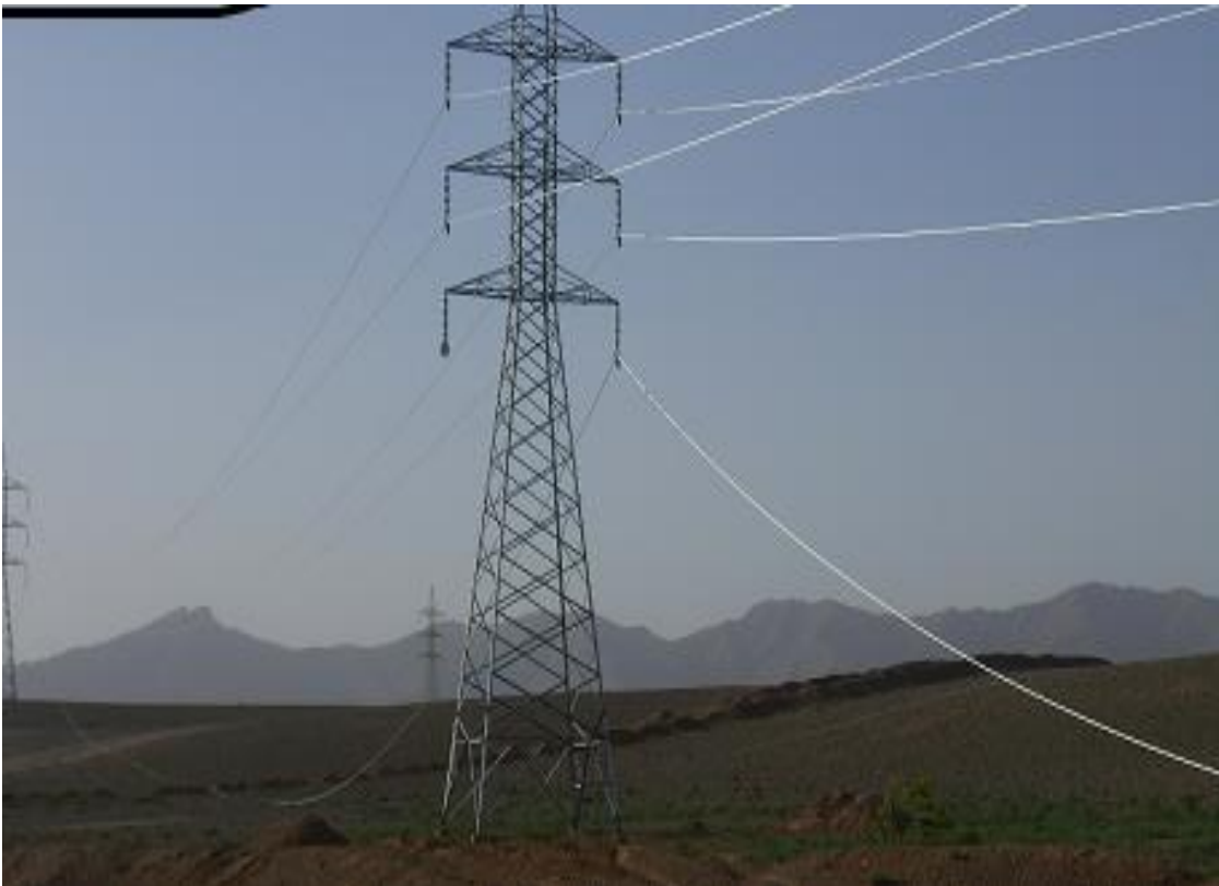
In and Out Double circuit stringing of new 132 KV T/L kalat – Mastung -- QESCO
