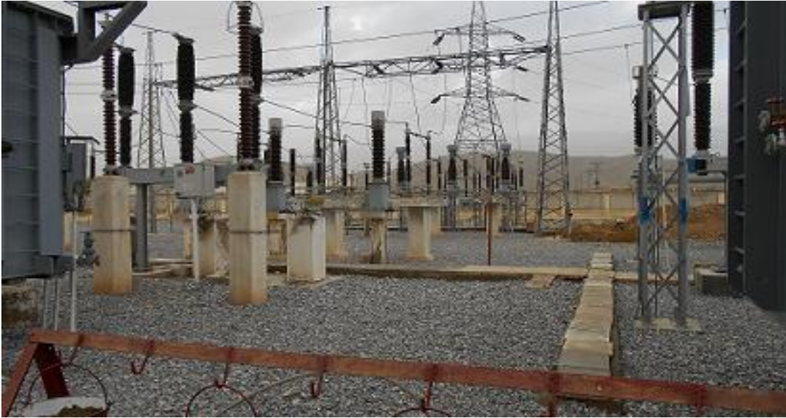
Transformer bay yard of proposed 132KV Grid station Muslim bagh – QESCO
